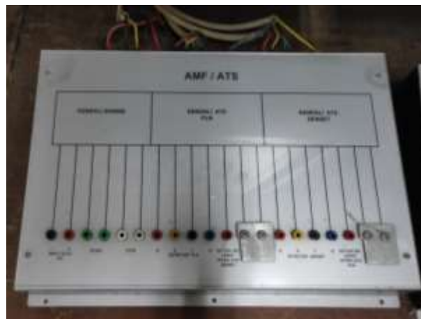
Gambar 7. Panel AMF ( Automatic Main Failure )
